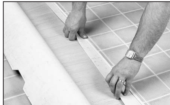
Fig. 19. Place a 2" (5.1cm) to 3" (7.6cm) scrap strip of flooring, face side down, centered under the seam.
