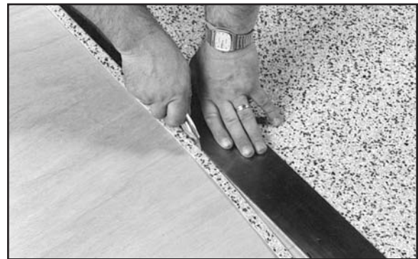
Fig. 27. Hold the utility knife at a 90° angle and cut a smooth, straight edge on the flooring.
