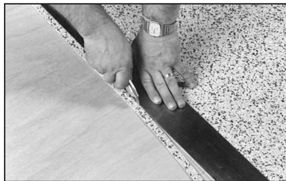
Fig. 1. Hold the utility knife at a 90° angle, cut a smooth, straight edge.
