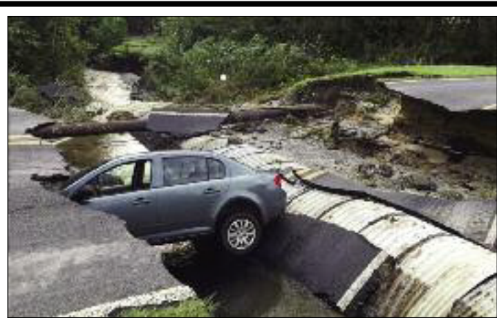
The aftermath of Hurricane Matthew has left many roads in disrepair, disrupting service deliveries for distributors in the Southeast.
